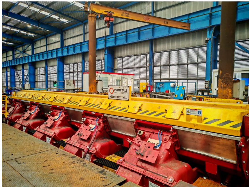
Newly installed Morgan Vee No-Twist Mill from Primetals Technologies at Celsa France's wire rod mill
