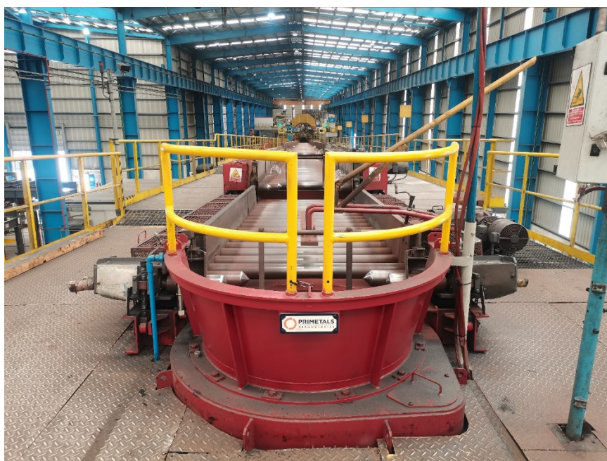
Newly installed Reform Tub at Celsa France's wire rod mill
