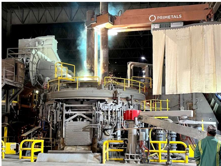
The first heat for NLMK Indiana’s 118-ton EAF after the modernization by Primetals Technologies.
